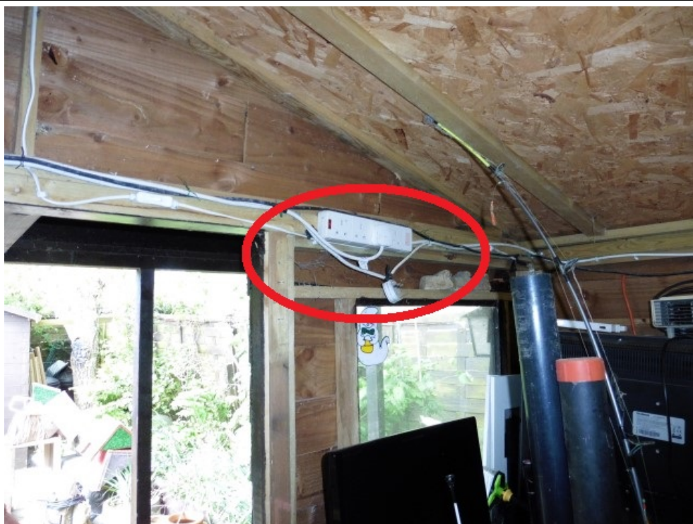
Poorly managed wiring in shed 4
