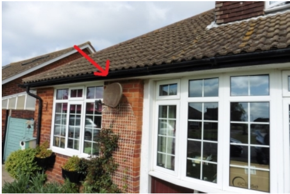
Sagging gutter at the front
