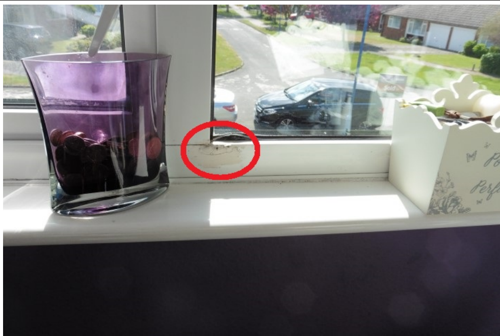
Damage to frame and seal in bedroom 1
