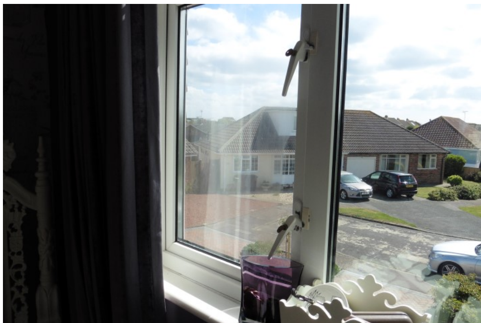
Bedroom 1 casement window panel blown
