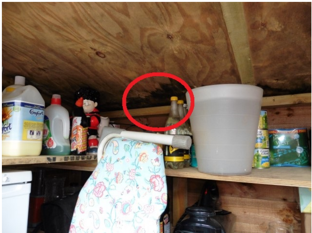
Staining on the underside of the roof of shed 2
