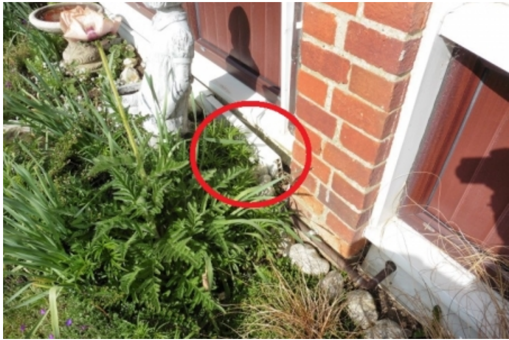
Loose plastic trim at the front
