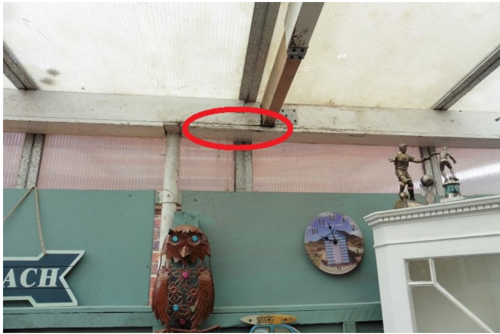
Possibly rotten timbers in the lean-to
