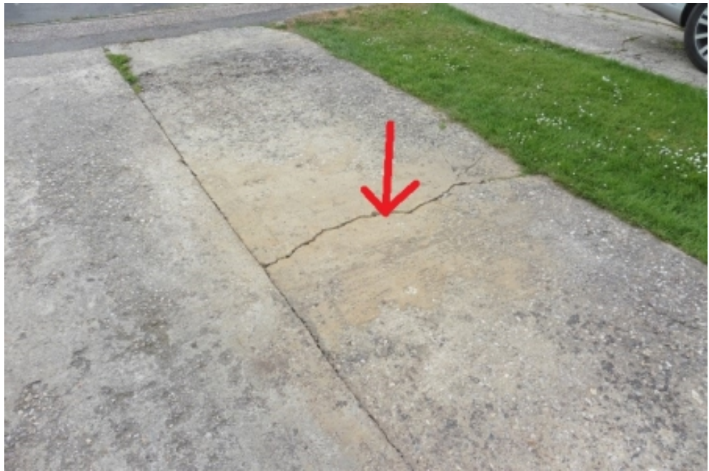
Cracking in the front drive
