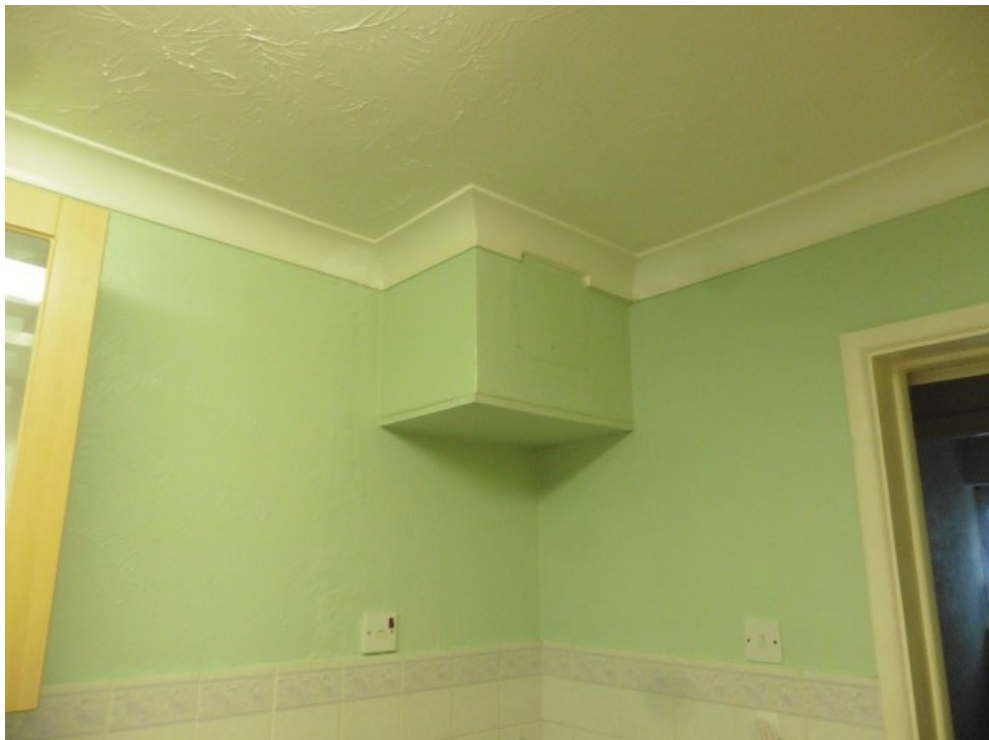
Right side chimney breast in the kitchen has been truncated
