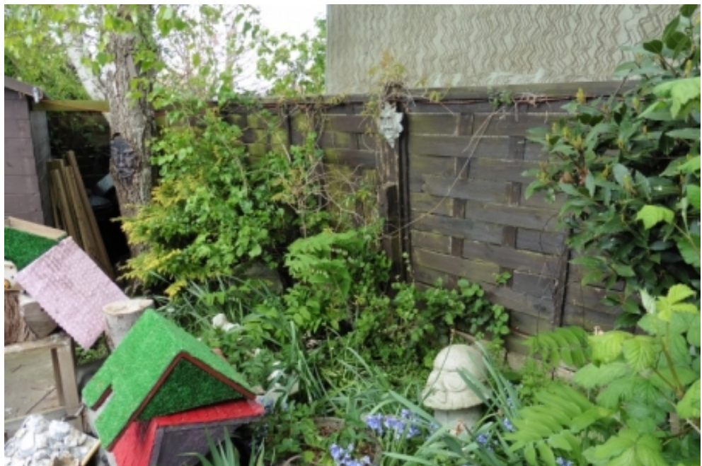
Rear boundary fencing maybe loose
