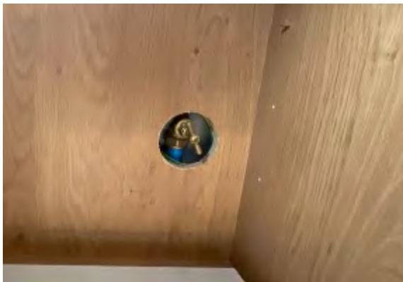
17. Water stop cock under kitchen sink
