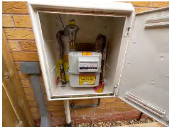
16. Gas meter cabinet
