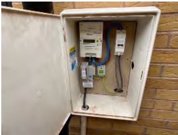
15. Electricity meter cabinet
